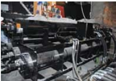
This bank of accumulators supplements pump flow so that the hydraulic power unit can deliver up to 600 gpm of flow during peak demand, even though the pumps are rated for a total flow of only 44 gpm.
